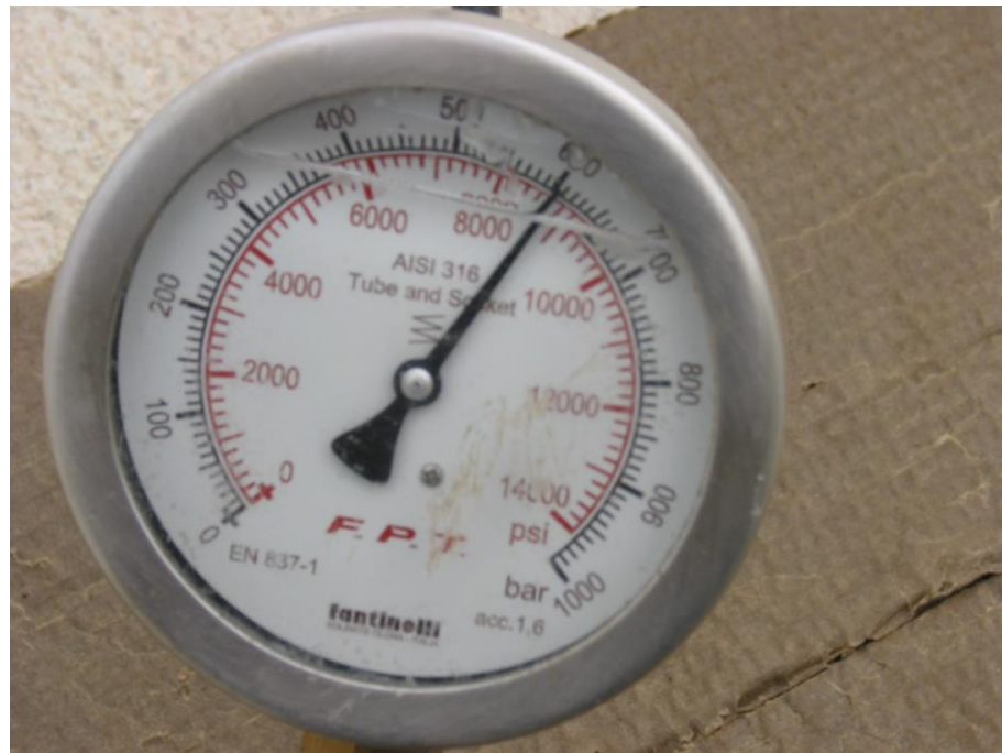
Fig. 4 Reading pressure gauge
